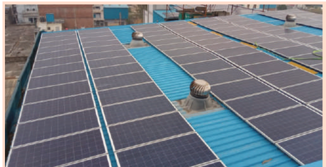
Capacity: 300kWp Location: Placero International Pvt. Ltd.(Sonipat)
