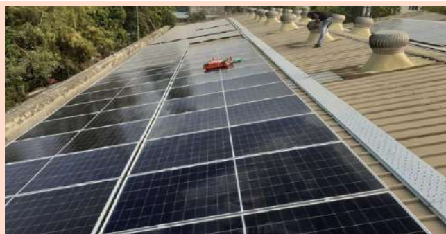
Capacity: 250 kWp Location: Radiant Chemtech Pvt. Ltd. Greater Noida, UP
