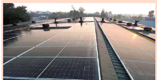
Capacity: 170kWp Location: Marvel Wires, Rorkee, UK
