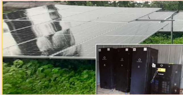
Capacity: 6MWh Location: Tripura
