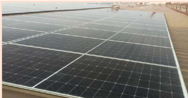
Capacity: 504 kWp Location: Awadh Rails, Haridwar
